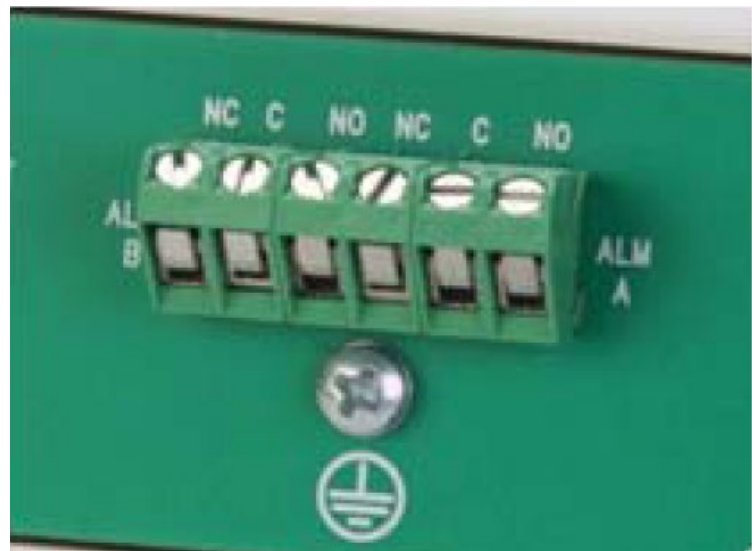
Fig. 7: Alarm Terminals on the Rear of the Panel
